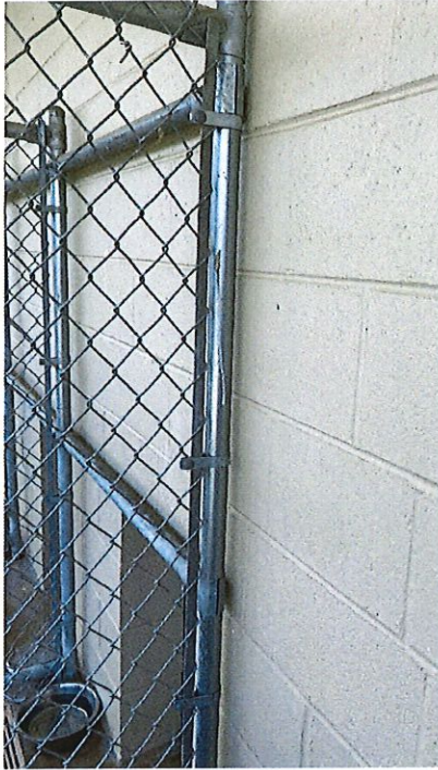
Unsecured chain link structure
